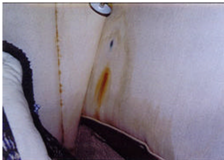
This is typical of the kind of interior damage that occurs from leaking deck joints.
